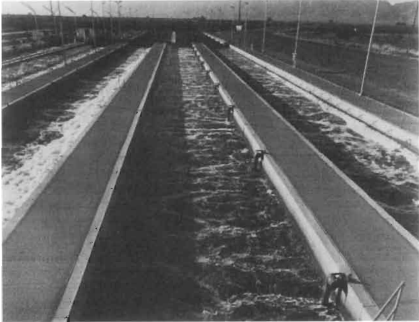
Figure 9-15. Activated systems with diffused aeration. (Photo courtesy of Envirex.)
