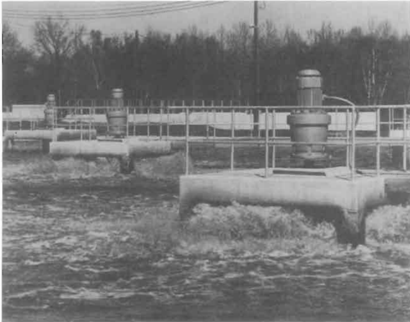
Figure 9-16. Activated systems with mechanical (surface) aeration. (Photo courtesy of Envirex.)
